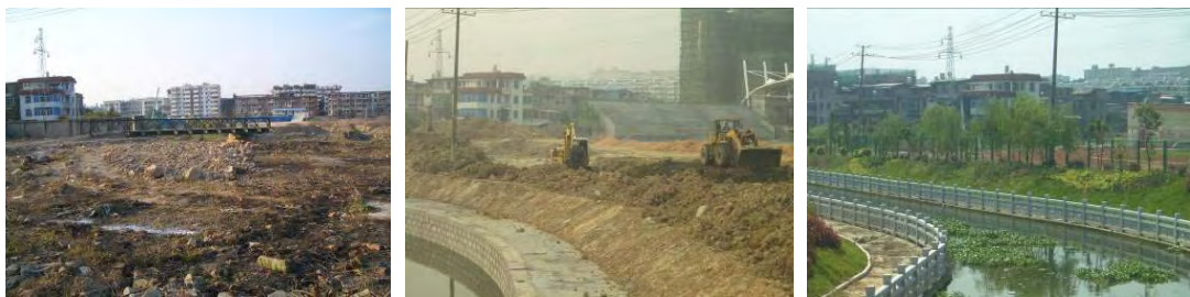
Comparison of the Yuejing River C1 contract in the vocational school before, during and after the rehabilitation
