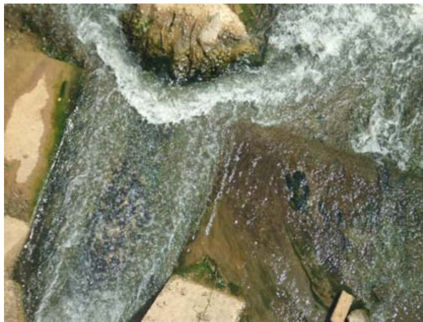
Fig.04: Water leaks through the Radial Gates of Mavilaru
