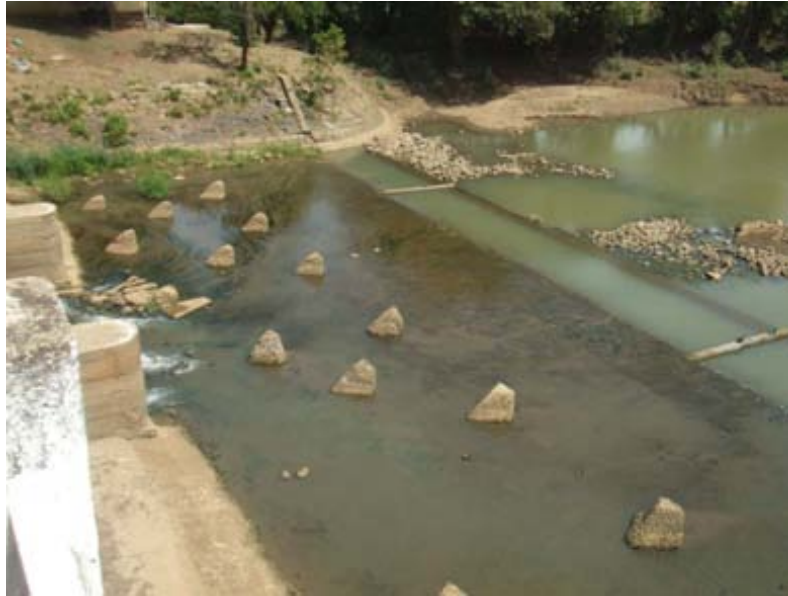
Fig.05: Water flow and leaks through the Verugal Anicut at Mavilaru
