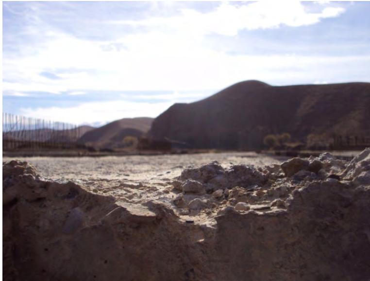
Figure 16 - Top surface of precast bridge girders do not appear to meet specified tolerances.
