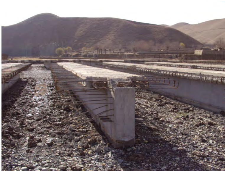
Figure 17 face of precast bridge girders do not appear to meet specified tolerances.
