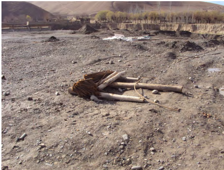
Figure 10 - Reinforcing steel is not stored as required by the specifications.
