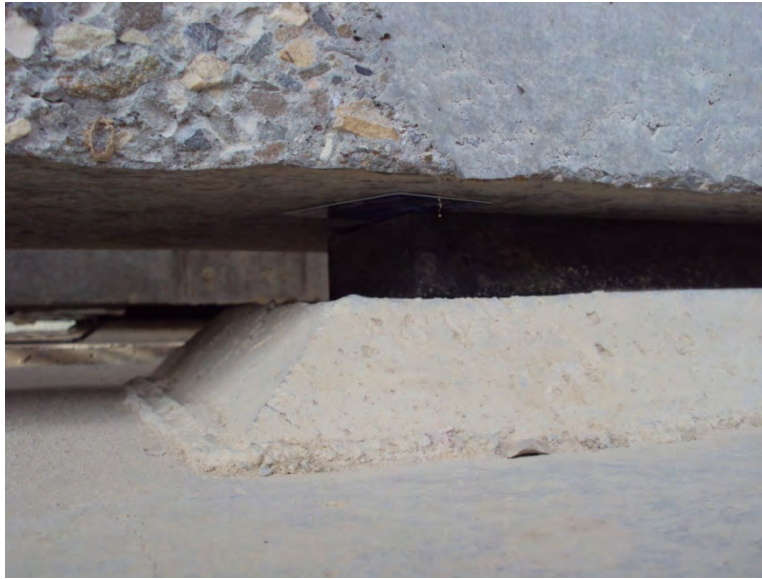
Figure 14 - Uneven bearing at Bridge 3
