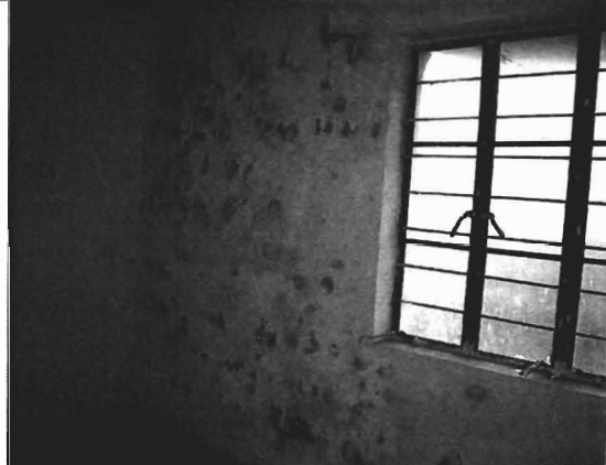
Damp in the wall of Block – A, Purba Putiari
