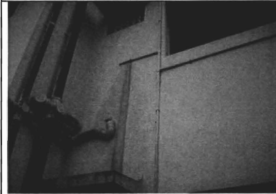
Leakage in water pipes - Purba Putiari
