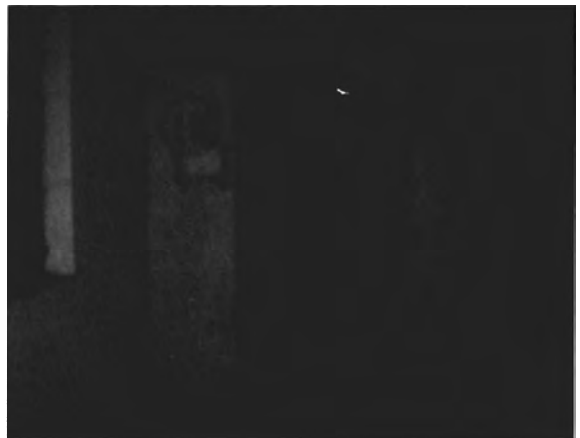
Picture shows water pipe is broken at Phase- iv
