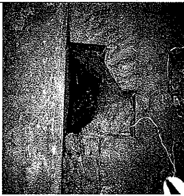
Leakage in water supply pipeline at Purba Putiyari R&R site
