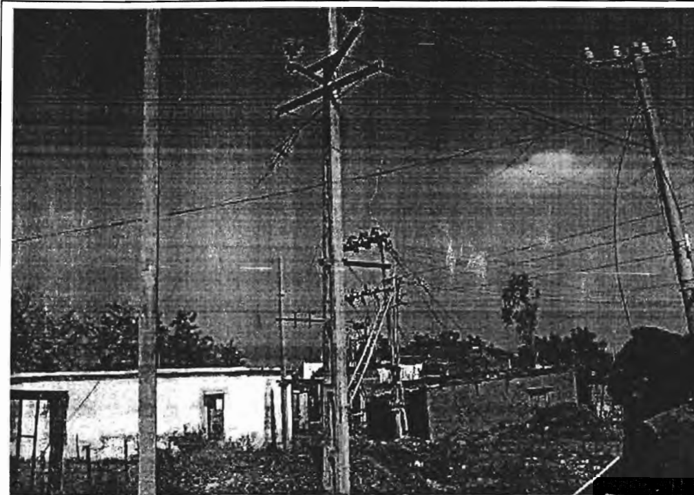
Utawad Sub-station – Line Separation
