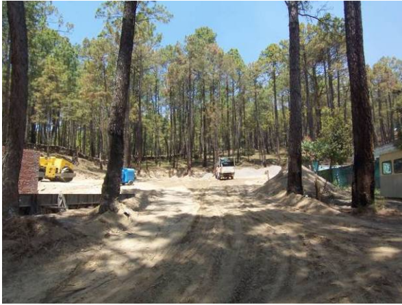
Fig.7: Water sprinkling on unpaved roads at construction camp site on Barechhina-Sheraghat Road (Contract VIII)
