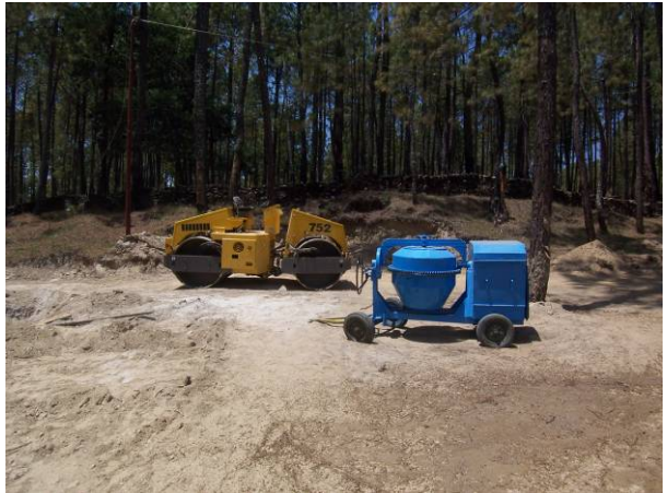
Fig.10: Site for storage of construction material at camp site on Barechhina-Sheraghat Road (Contract VIII)
