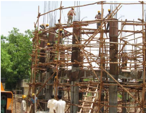
Photo 3: Column casting - utilisation of PPE like helmet, safety belt noted at Alwar
