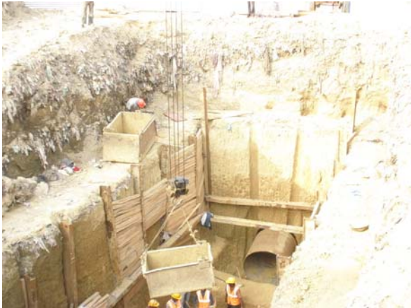
Photo 1: Safety arrangement – Waste water Package at Tuleda Road Alwar
