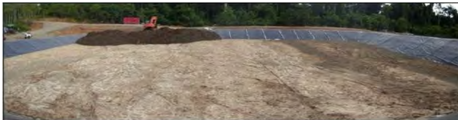
Figure 5. New Organic Waste Landfill
