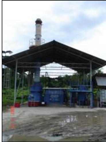
Hazardous Waste Incinerator
