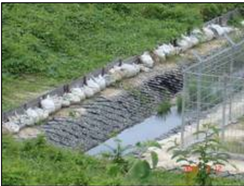
Permanent Drainage at the Shore Base Area
