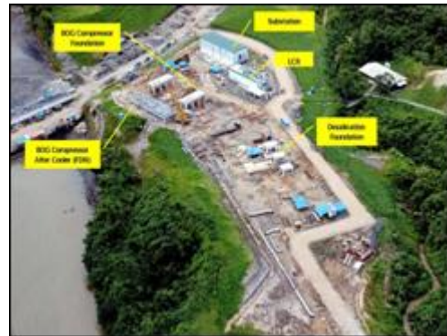
BOG Compressor & Desalination
