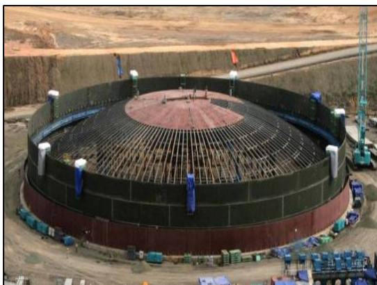
Tank – 1 as of end of October
