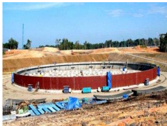
Tank – 2 as of end of October
