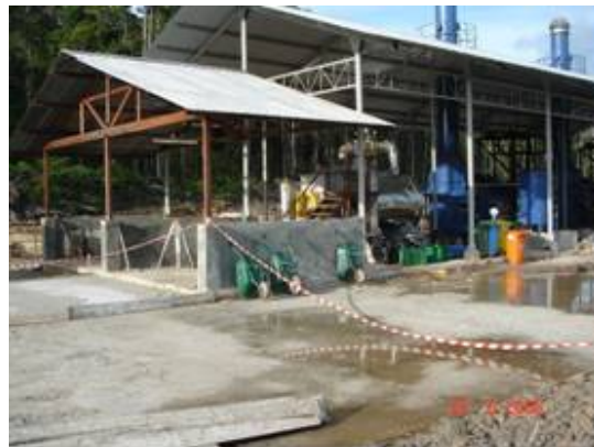
Non Hazardous Waste Incinerator
