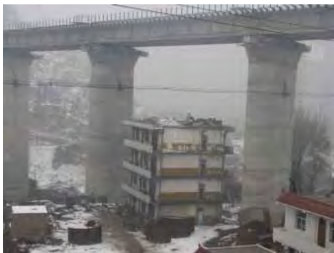
Picture 7: A residential building under Taizhongyin Bridge, which has been cut for demolition purpose because of the construction of Tai-Zhong-Yin Railway in Liulin County, Lvliang, Shanxi Province
