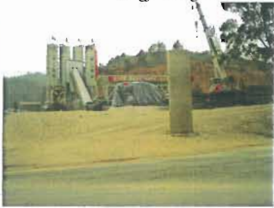
No. 9 mixing station (K148+000)
