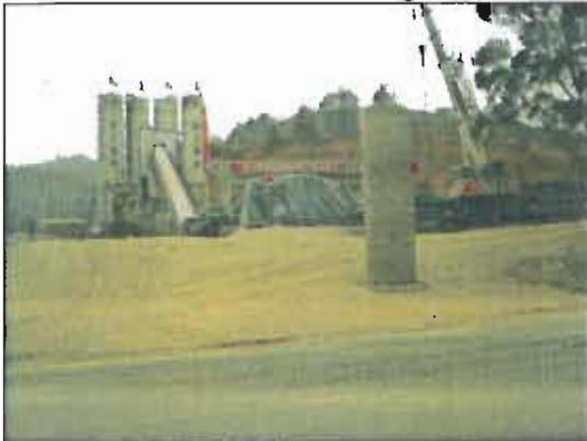
No. 9 mixing station (K148+000)
