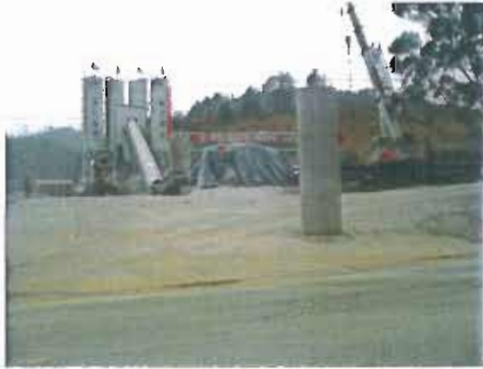
No. 2 mixing station (K148+000)
