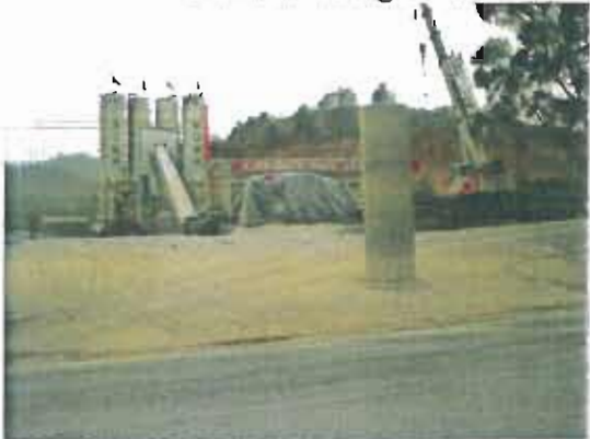
No. 9 mixing station (K148+000)
