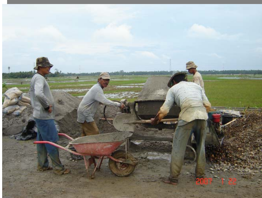
Figure 4: Four WUA's members in DI Krueng Tuang, Aceh Utara is "gotong royong " using a concrete mixer to prepare required materials needed to complete construction of tertiary canals
