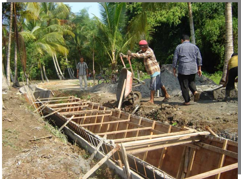
Figure 2: A member of Water User Association (WUA) in DI Alue Ubay, Aceh Utara is actively constructing their own secondary canals. Usually, the Secondary canal is constructed by professional contractors
