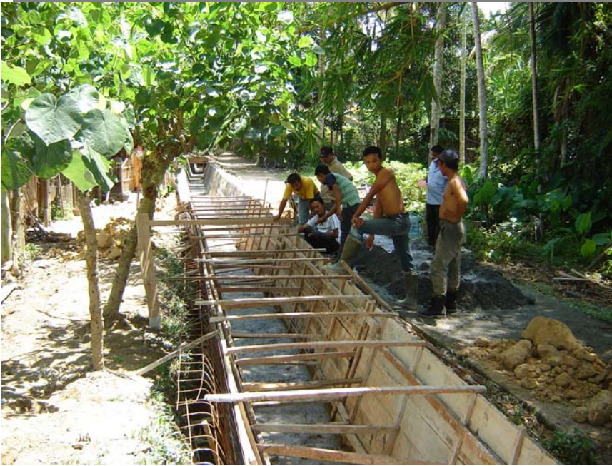
Figure 3: A Field Staff of B & V Consultant , Koordinator Tenaga Pendamping Petani (KTPP), is providing a technical assistance to the members of WUAs during the construction in DI Alue Ubay, Aceh Utara
