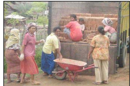
Women's participation in building their own houses – community contract scheme in Seuneudon. Photo: Adhitya Palgunadi
